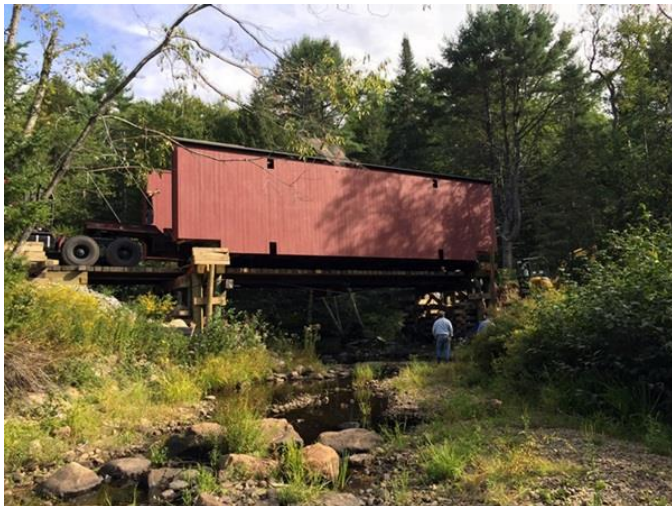
After being backed across a temporary bridge, the covered bridge will be jacked into location once that temporary structure is removed.
